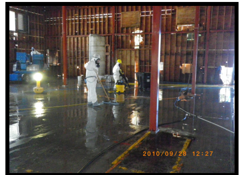
Steel & concrete cleaned w/ pressure washers / water capture with shop vacs to storage tank
